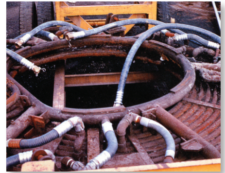
Circulating water in an electric arc furnace cooling roof or furnace door.
